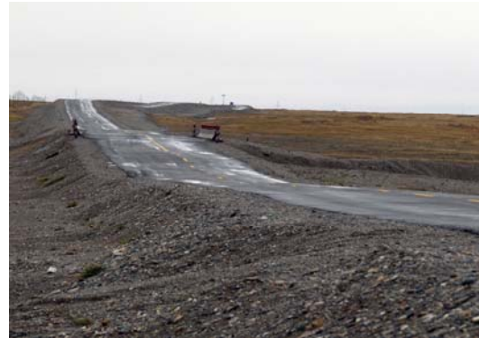
Figure 1. Example of the damage of a road embankment in the high altitude Qinghai-Tibet region due to uncontrolled permafrost melting (source: http://nsidc.org/frozenground/people.html ).
